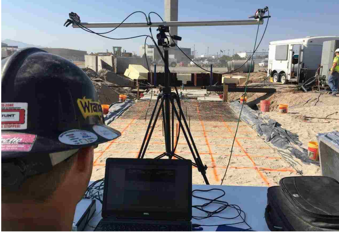
Figure 3-9: DIC cameras on tripod just past the north edge of the backfill
